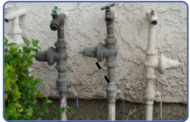
The master valve to a condominium or apartment may be more difficult to locate because several may be grouped together.
